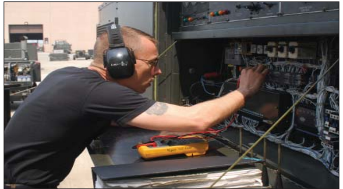
Tech. Sgt. Heath Warren trouble shoots an MA3D air conditioner which is used to cool the avionics section of air craft here.
